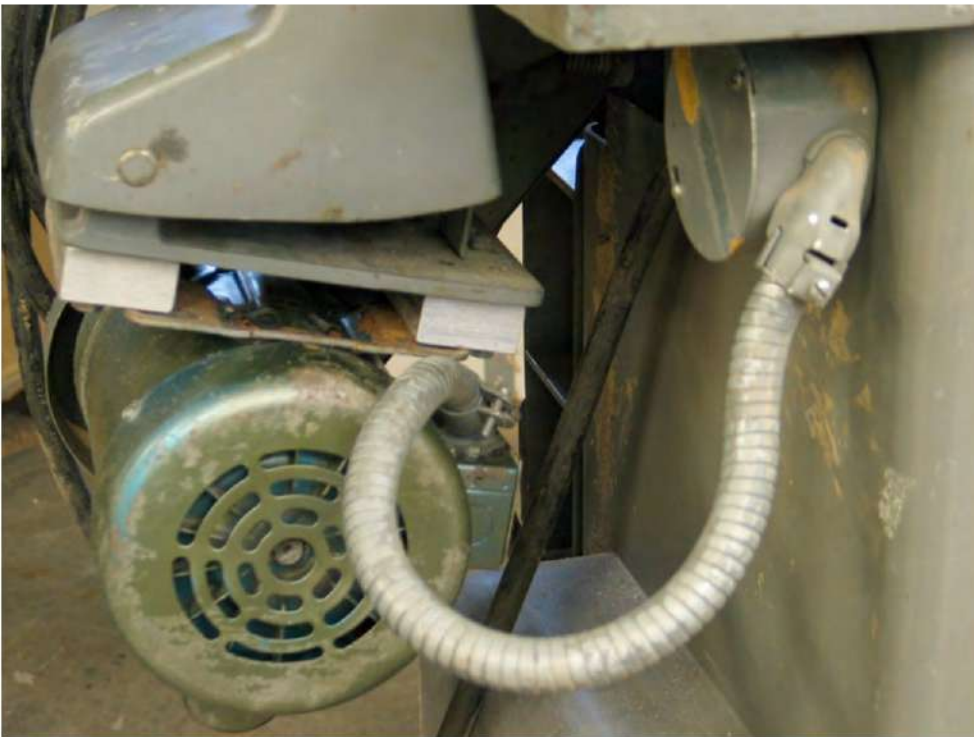
Figure 49 The 56 frame, 3450 rpm motor installed
